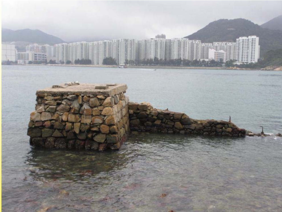
礦場西端碼頭及圍牆 Quay and Retention Wall at the western end of the site
