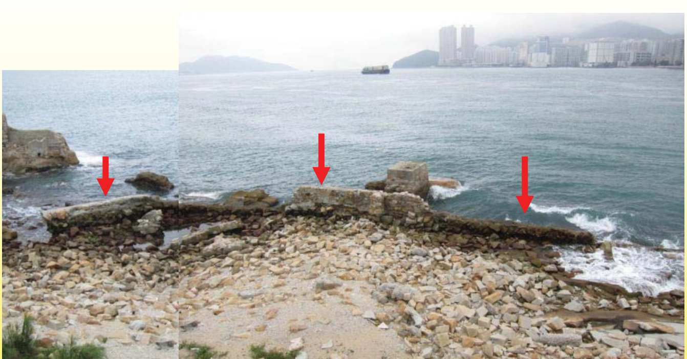
礦場南邊碼頭及圍牆 Quay and Retention Wall along the southern boundary of the site
